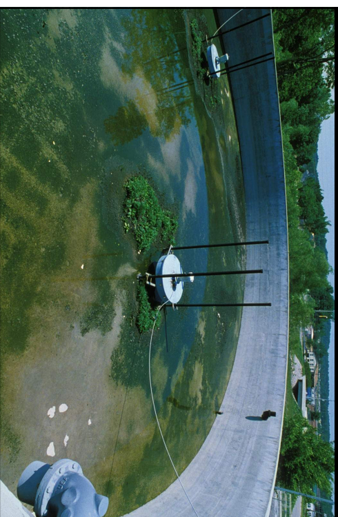
Equalizing Dry Pond to Control SSO Problems, Moody, AL
