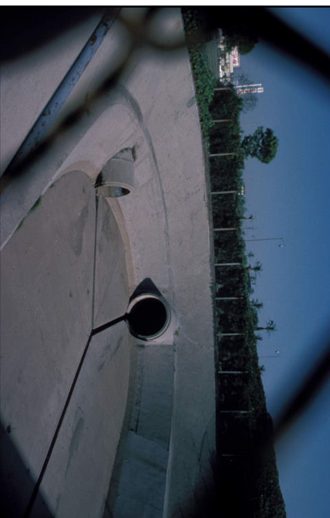
Dry Detention Pond Forebay for Stormwater Pump Station, Los Angeles, CA
