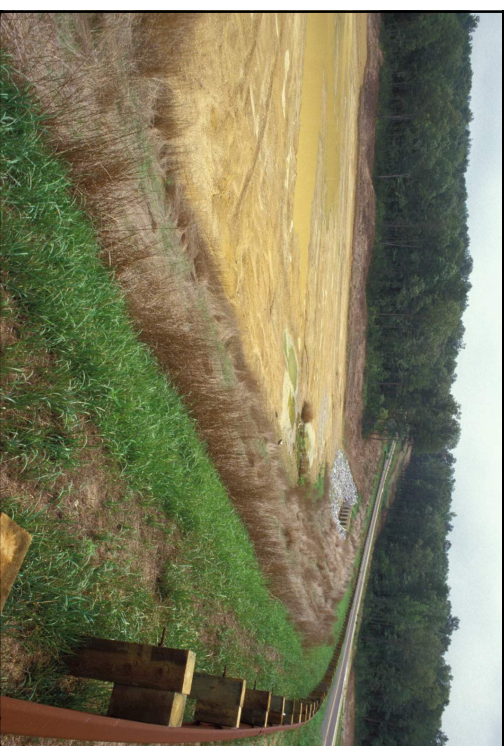
Wet Ponds Located in Areas of Karst Geology may have Sinkholes
